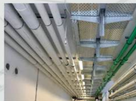
Aqua-Plus Pipes & Aqua-Plus Prins in 5* Hotel compound
